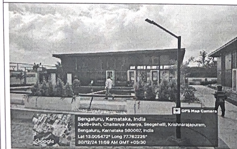
Partly civil & metal structure at Southern side of the apartment, still present.
