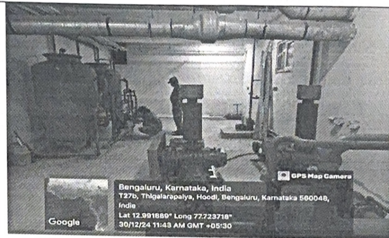
STP MBR Tank adjacent to Aeration tank
